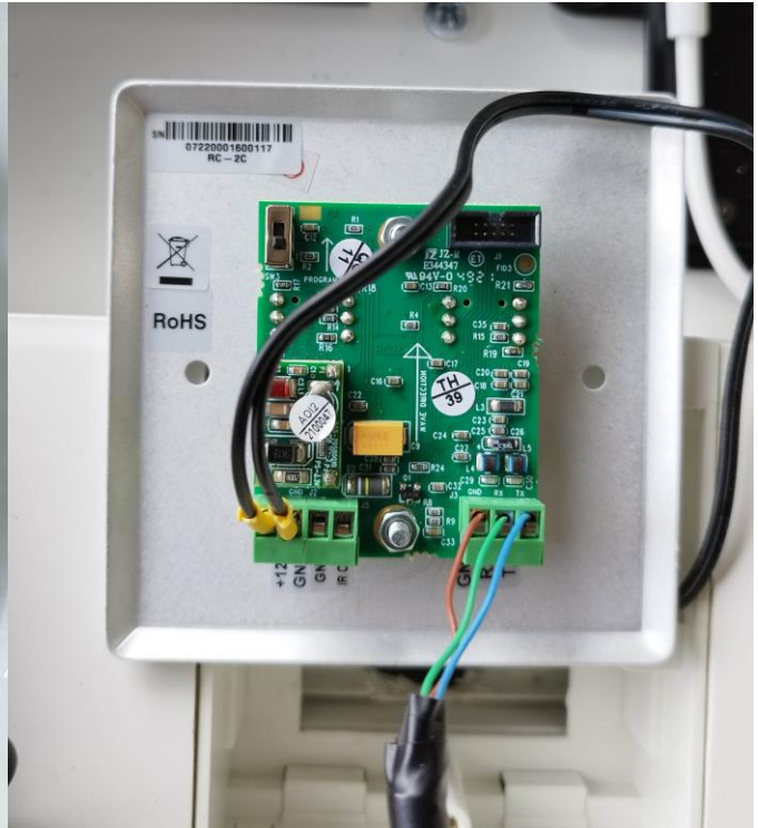
Wiring for projector controller
